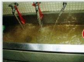
▲取付前の蛇口部の赤水 Before installing (rusty water from the tap).
