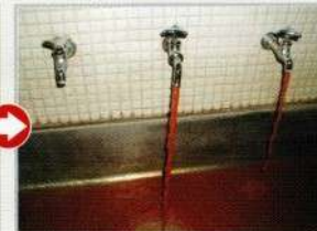
▲取付直後の蛇口部の赤水 After installing (red rusty water from the tap).
